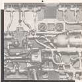
HYDRAULIC SYSTEM FILLERS, ACCUMULATOR AND PRESSURE GAGES
